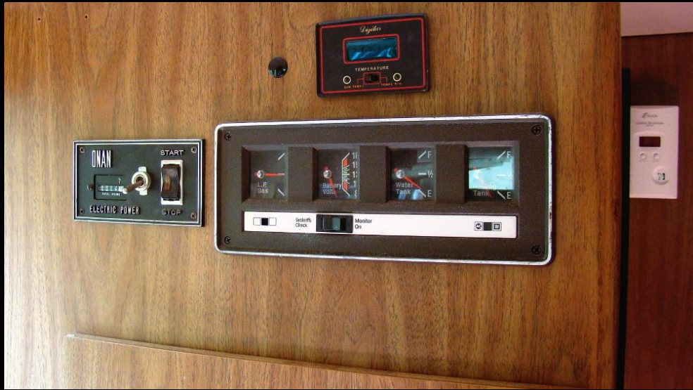
Added gauge to show refrigerator temperature
